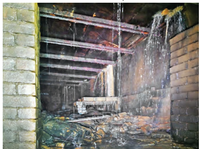
Abandoned adit showing the amount of water draining down into the tunnel. Photo Gerald Tompsett
